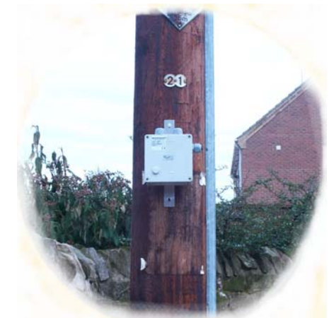
Pole mounted M61
